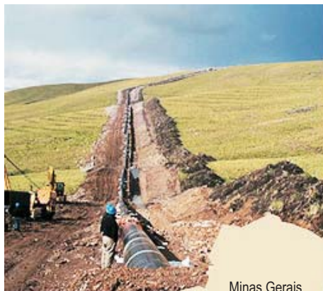
Building a 525 kilometer pipeline through the topographically varying landscape is a demanding job.
