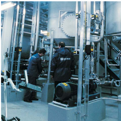
The detailed, error-free and continuously updated information of the 3D model greatly improves the installation phase
